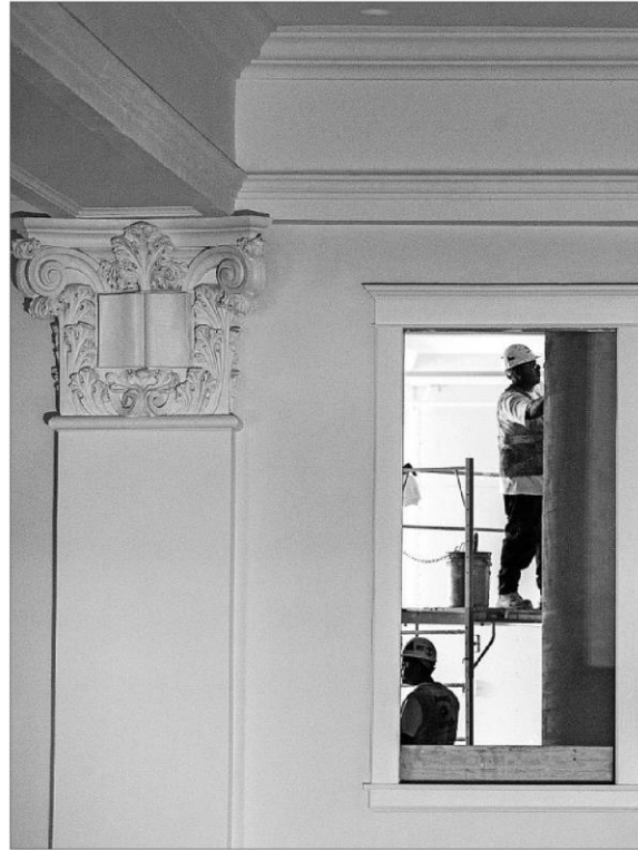
Original molding and details adorn the building's interior, where crews continue the renovation.
